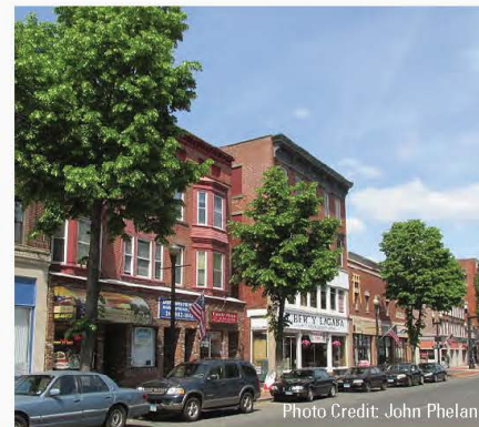
Reconstructed West Main Street sidewalks from Cook Avenue to South Grove Street.
